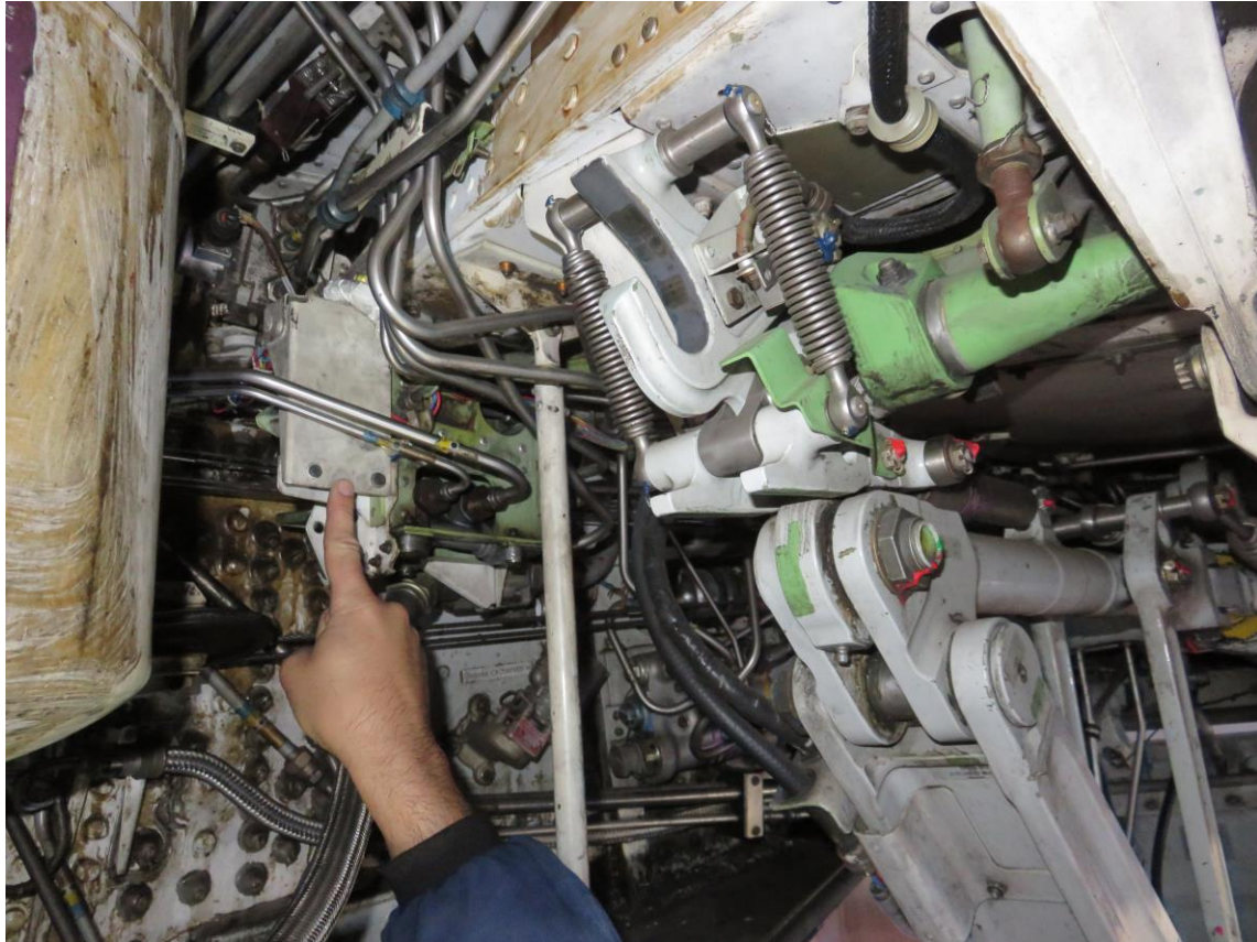
Figure 7: The Air/Ground proximity sensor pointed out in the right main wheel well.
